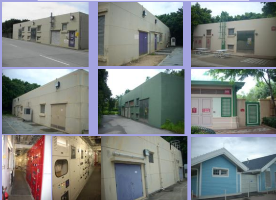
Electrical Installation - Substations
