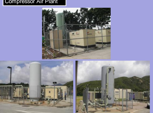
Compressor Air Plant
