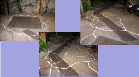
Marking of new cut line on concrete floor to match the Theme
