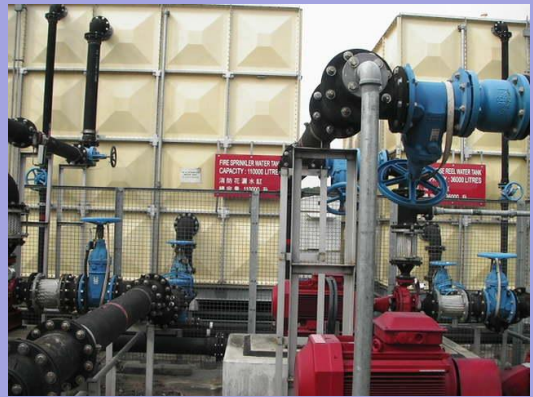
Fire Service Pumping Installations
