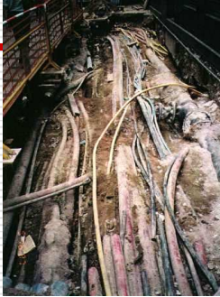
A congested trench at Tsun Yip Street, Kwun Tong
